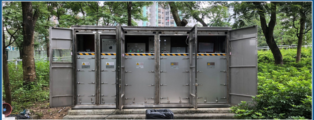
Floodgate installed at Highway lift pillar box
