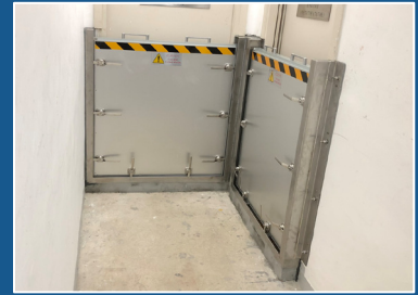
Two floodgates installed together in Flushing Water Tank and Pump Room
