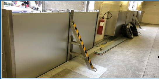
Double panel floodgate with water prevention hoods installed at CLP Power Substation
